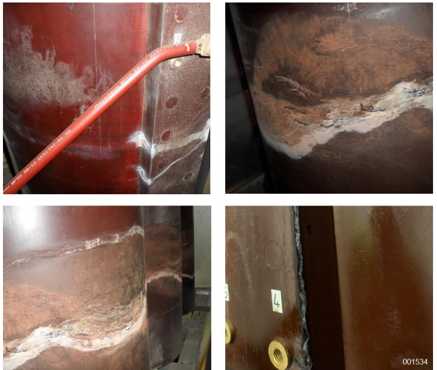
Fig. 24: Traces of creep current and partial discharge traces
